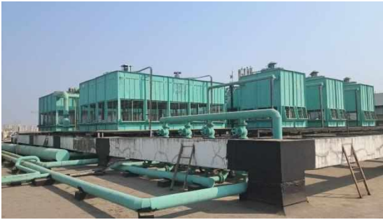
View of Cooling Towers at Subject Project
