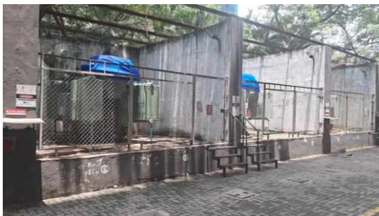
View of Transformers in Subject Project
