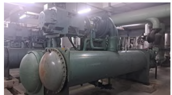
View of Chillers in Subject Project
