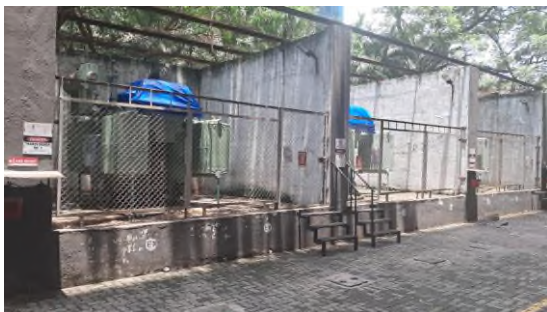
View of Transformers in Subject Project
