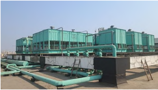
View of Cooling Towers at Subject Project
